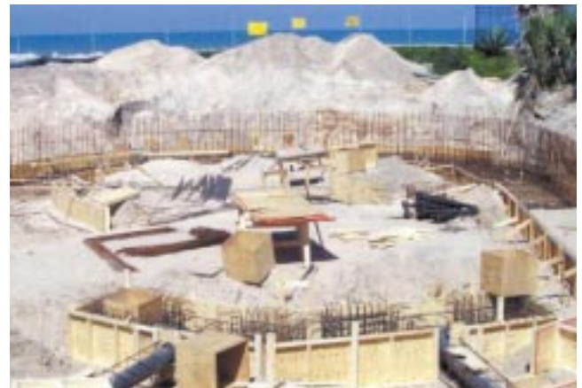
Lockwood Greene chose MMFX over traditional alternatives for the dolphin and sea life lagoon at Marineland of Florida after determining that MMFX, in conjunction with standard concrete cover practices, would result in an up-front savings of 8% .
